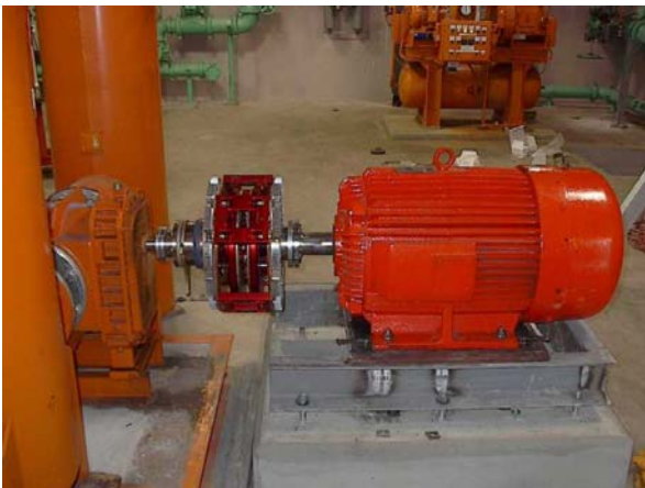
Figure 1- MagnaDrive ASD installation in Port Angeles
